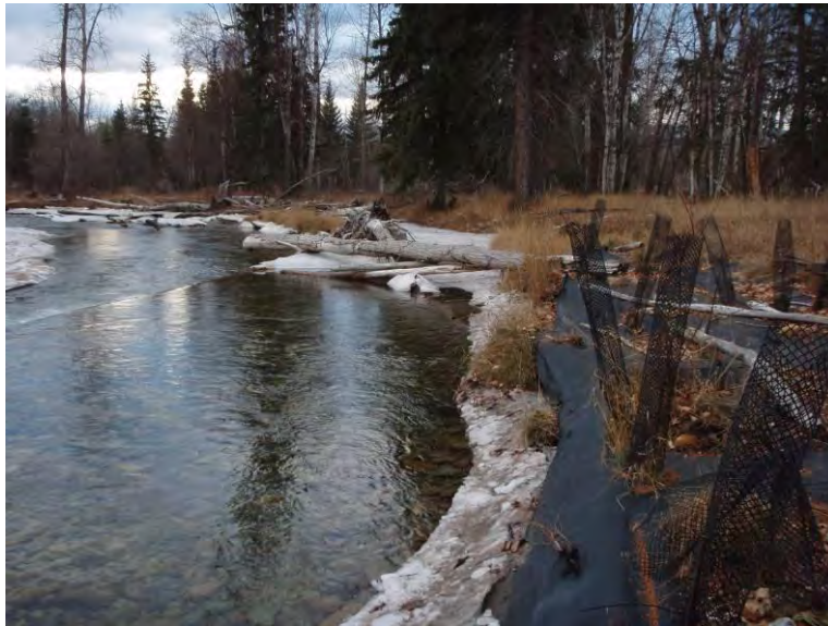
Figure 11. Photograph of Fall 2005 planting site. Photograph shows the extent of lateral erosion that occurs on outer banks within the reach. The black plastic weed mat was placed approximately three feet from the edge of the stream bank in 2005 and in December, 2007 one and a half feet of weed mat had slumped into the channel, indicating at least four feet of lateral erosion occurred along this bank.
