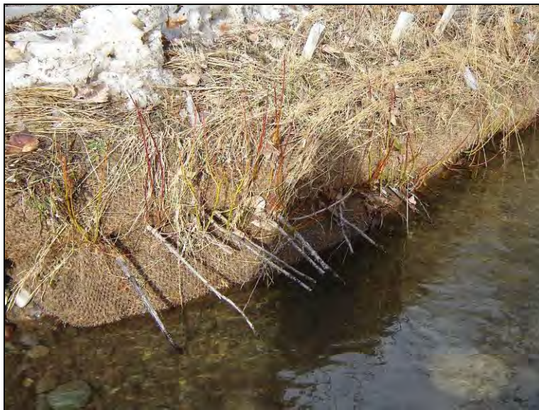
Figure 19. Toe scour and slumping of soil lift installed in 2005, but new willow shoot growth on decadent stems and good herbaceous cover of seeded species on top lift.
