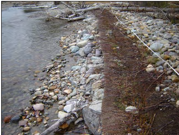
Figure 16. Photograph showing how tape is laid across top layer of soil lift to record data in five-foot increments.
