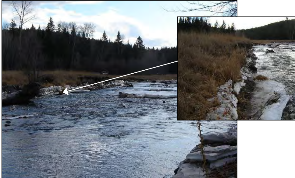
Figure A-14. Photograph showing area selected for set back treatment. Inset photograph shows vertically eroding bank.
